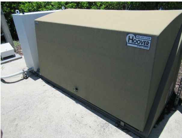
Irrigation pump station
