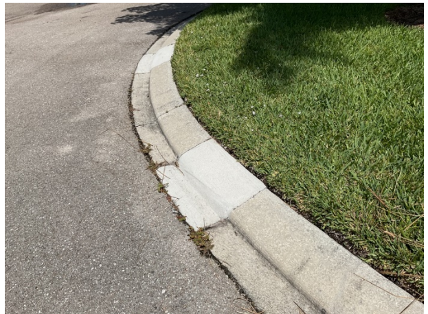
Previous repairs on concrete curb
