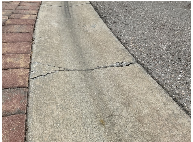
Concrete gutter cracks
