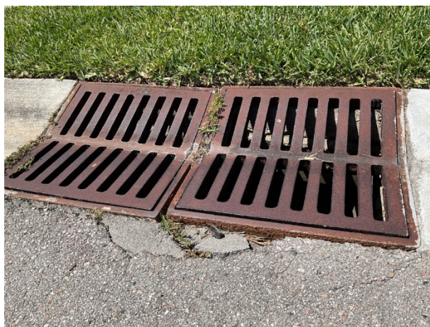
Pavement damage near catch basin
