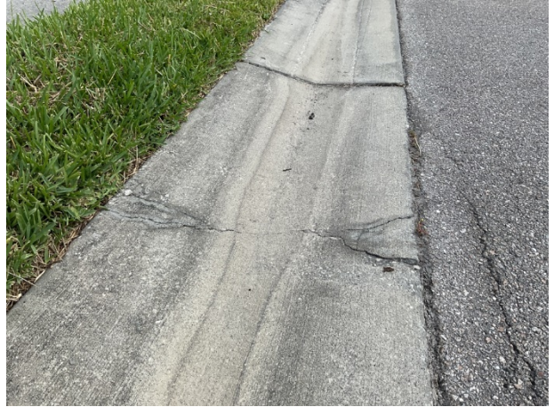
Concrete gutter cracks
