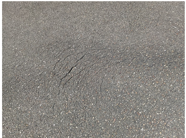
Pavement slippage at the Cypress Shadows Boulevard
