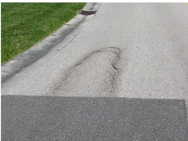
Pavement slippage at the Cypress Shadows Boulevard
