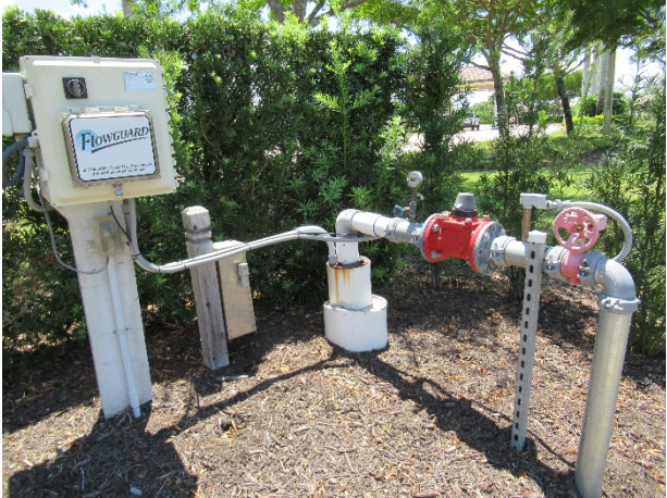
Well pump and control
