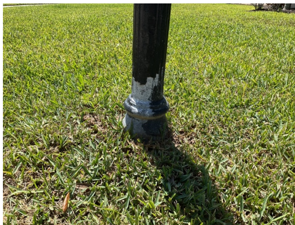
Sign finish deterioration
