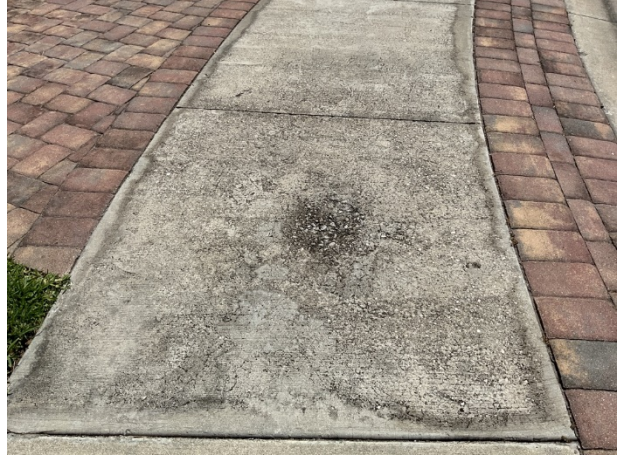
Concrete sidewalk damage
