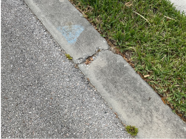
Concrete curb damage
