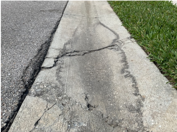
Concrete gutter damage
