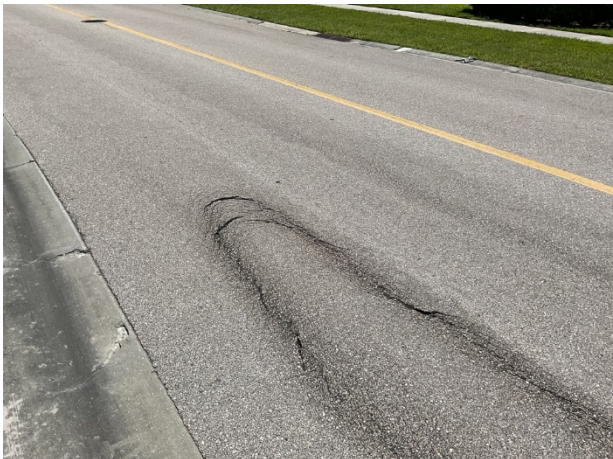
Pavement slippage at the Cypress Shadows Boulevard
