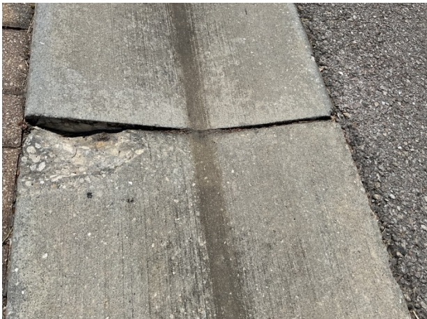
Concrete gutter damage
